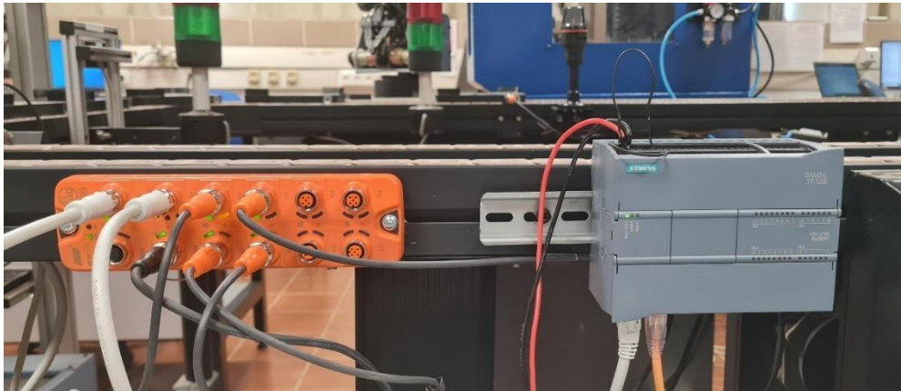
An IO-Link master and S7-1200 controller mounted onto the SmartCIM conveyor
